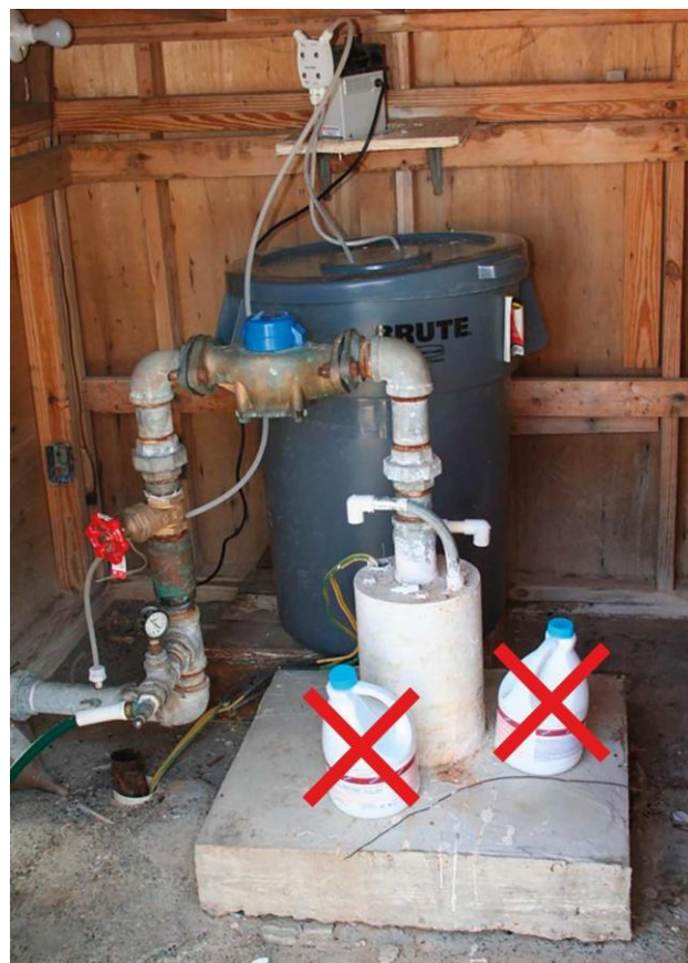
Figure 51 - Wellhead with pad in a well house. If this well needs to be serviced, the roof of the well house will need to be removed to allow space for an overhead crane or winch to remove pipes and the pump from the well. Also, the two bottles of chemicals should not be stored in the well house, and the well owner should not self-chlorinate their well (photo credit: G. Schindel).
