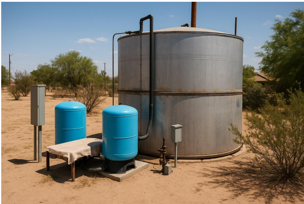
Figure 25 - A shared well system with above-ground storage and two bladder pressure tanks delivering water to two households.
