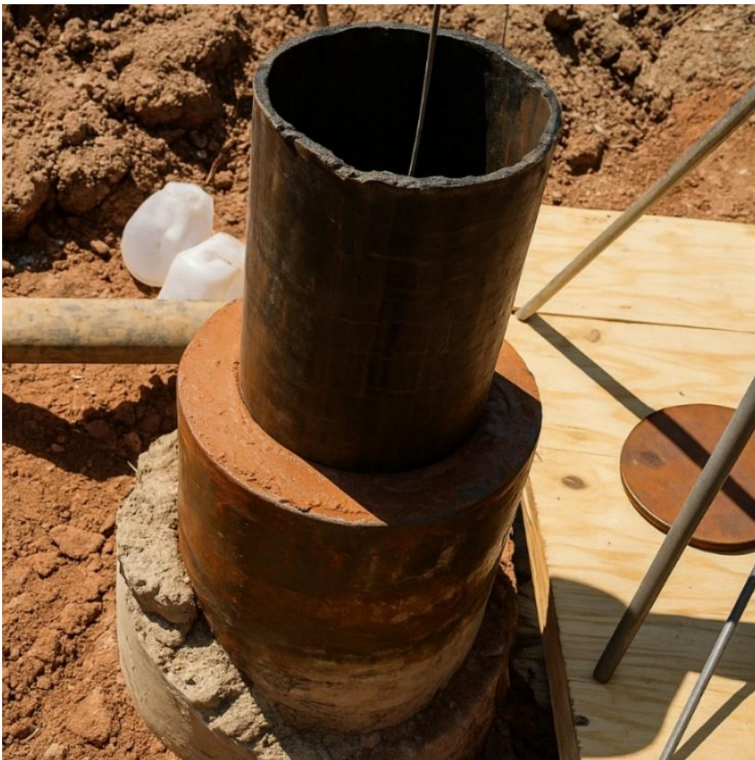
Figure 17 - Photo of sanitary seal grout in the annular space around the surface casing of a well prior to the construction of the concrete apron.
