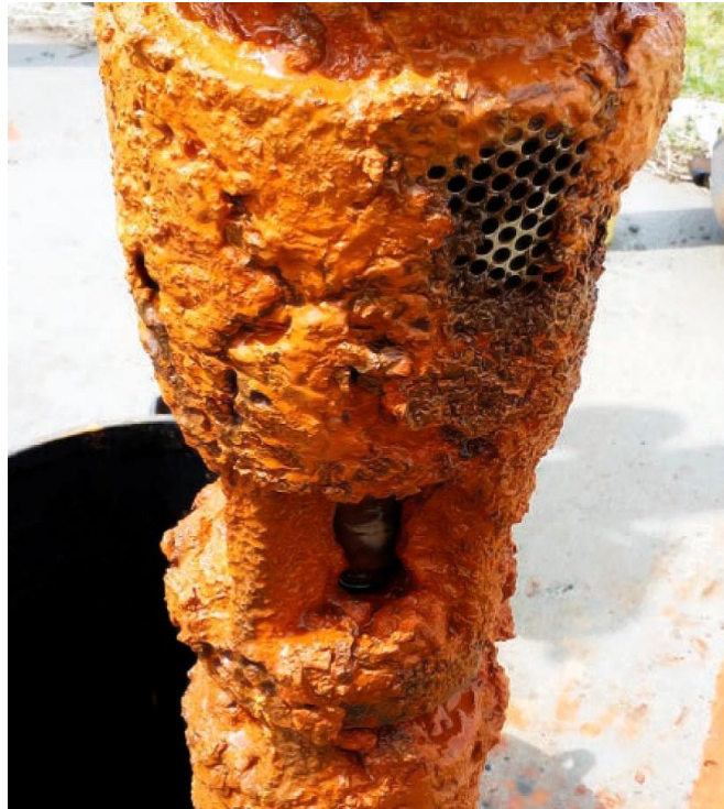
Figure 30 - Buildup of biological slime and mineral crust on a submersible pump inlet (photo provided by the National Groundwater Association, NGWA, for Artiola & Uhlman, 2017).
